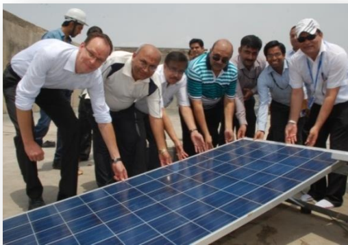
Construction of 500 kW begins at Dwarka Sector-21 Metro Station; GIZ and DMRC officials seek blessing
